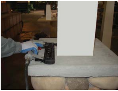
10) Nail column to post ONLY ON THE BOTTOM . Do not attach at center or top (to allow for expansion).
